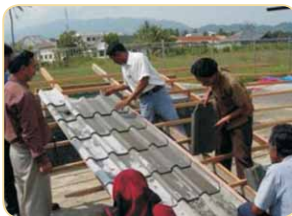
Training of masons for MCR tiles roofing installation at Banda Aceh, Indonesia
