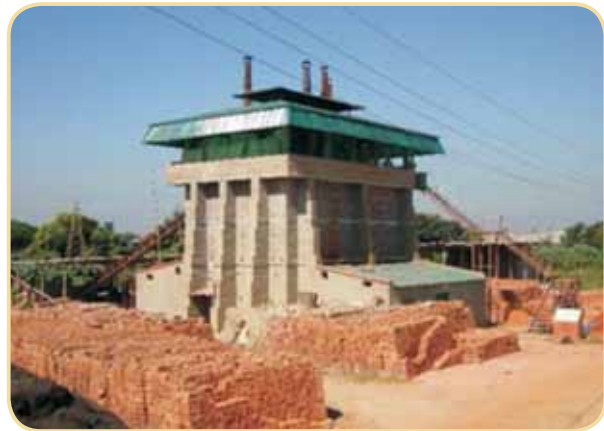
Energy efficient brick kiln technology in Bangladesh
